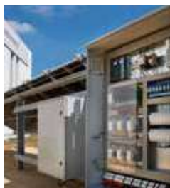
Pv Solar Test Lab
